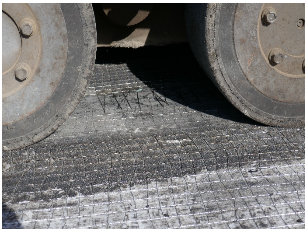
Figure 19: Shift caused by the asphalt paver's long period of standstill
