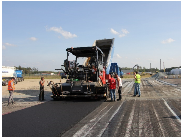
Figure 6: Installation of the top layer with a Vögele SUPER 1803-3i asphalt paver
