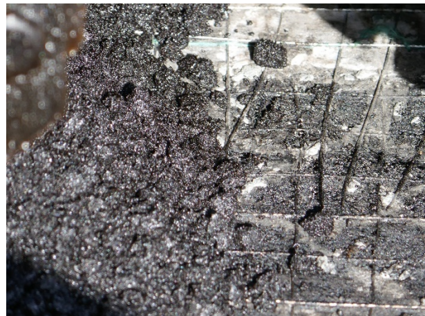
Figure 20: Shift caused by the asphalt paver's long period of standstill
