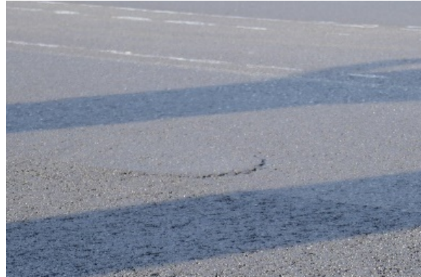
Figure 22: Planned defect in the top layer caused by the lack of bonding due to the Teflon sheet
