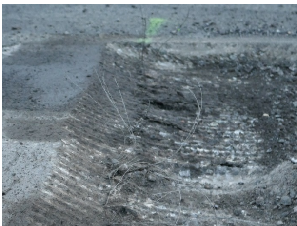
Figure 29: Milling edge with longer steel cord
