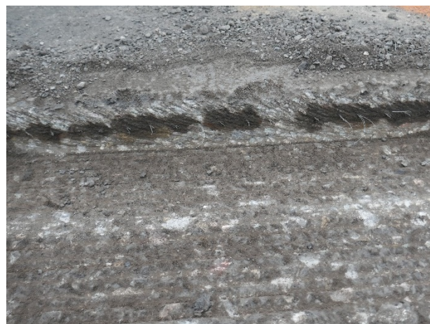
Figure 30: Milling edge with torn steel cord
