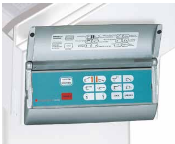
Emergency operating panel: the second control system can be activated through the integrated emergency operating panel.
